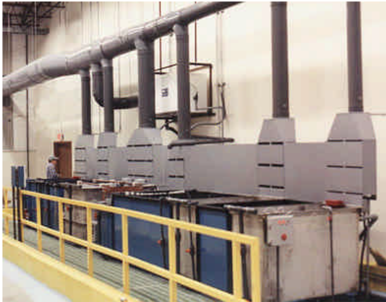
FIGURE 5A. Twelve-station line with 350-gallon electropolishing tank, ventilating system, evaporative recovery system, and semi-automatic waste treatment unit. The space occupied by the line is approximately 10 feet wide x 35 feet long. The ventilation system is designed for approximately 10,000 cfm. The line produces superior quality electropolished parts for semi-conductor and pharmaceutical applications.
